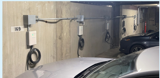
Figure 1. Ten chargers (Level 2) installed at above property for <$3,000 per charger
